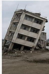
Liquefaction-induced building tilt
